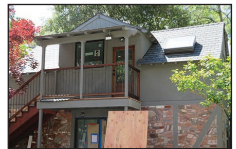
KATHY ENZERINK An accessory dwelling unit is under construction on Moraga Way.
