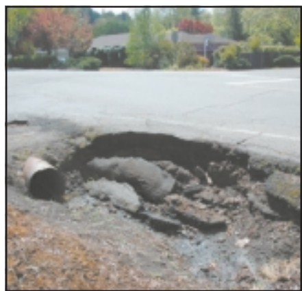
PAT RUDEBUSCH This pothole at Hillcrest and Overhill shows the deterioration of the roadway and culvert.
